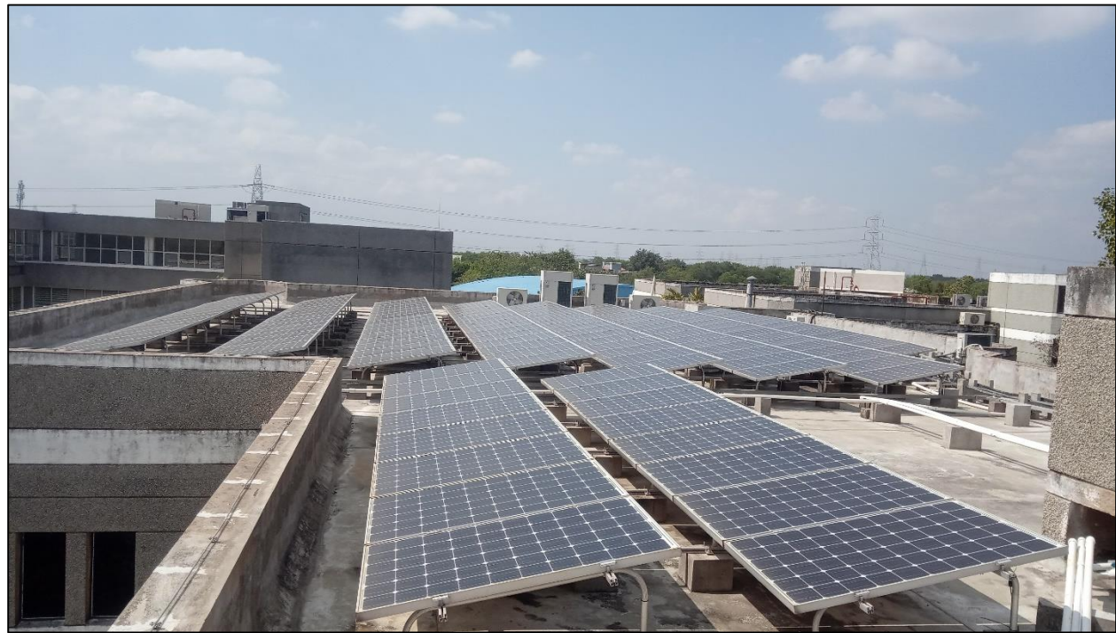
Solar Panel Installed at Admin Block of the campus.
