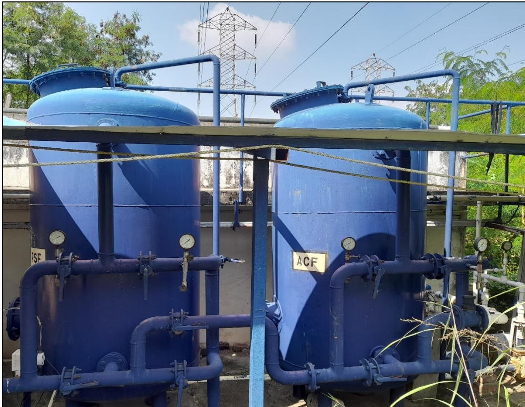
Pressure Sand Filter and Activated Carbon Filter at STP
