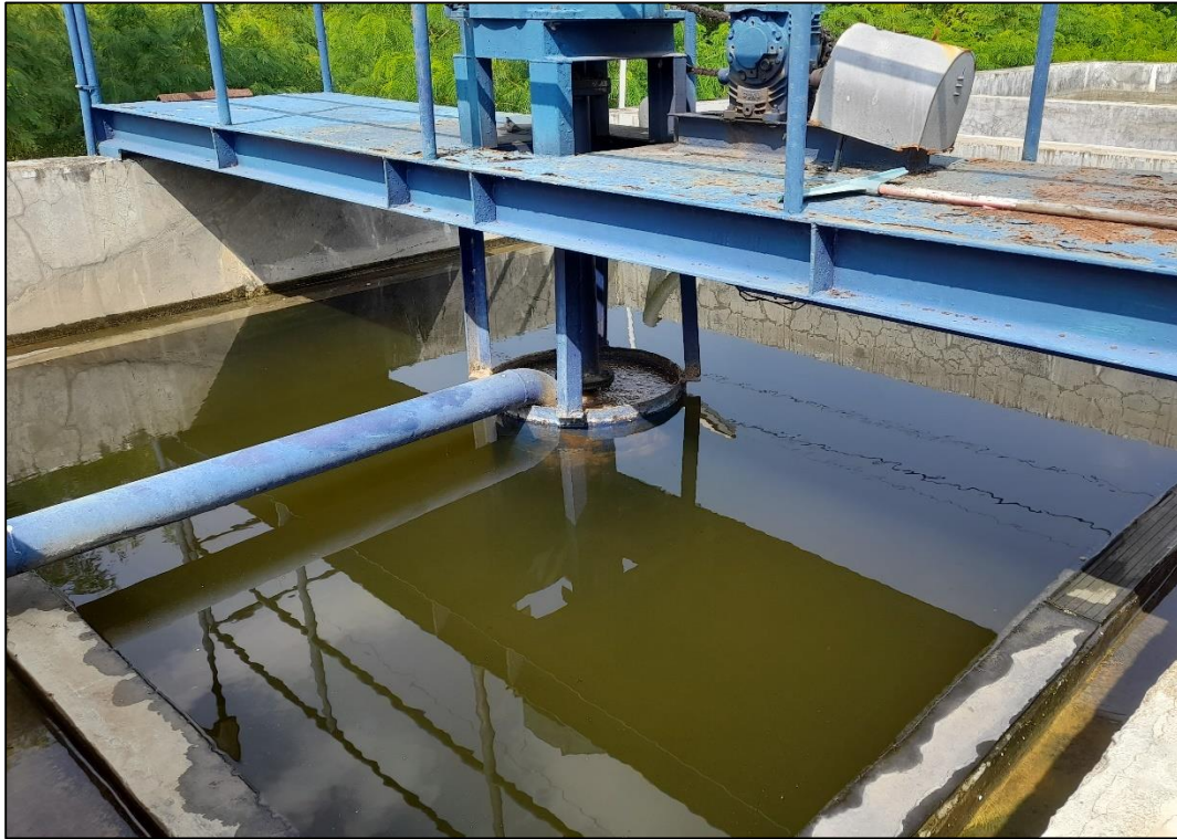
Clarifier Tank at STP
