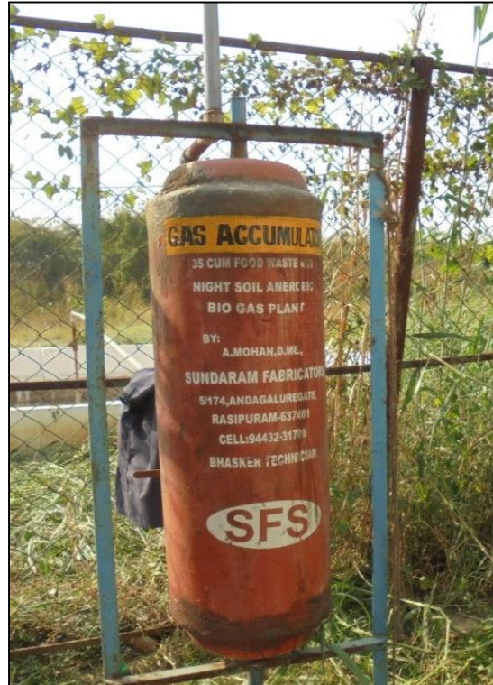
Gas Accumulator at Bio Gas Plant
