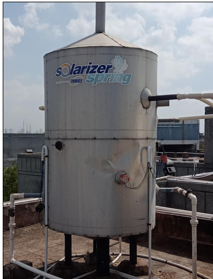
Water Heater installed at Gents and Ladies Hostel Blocks
