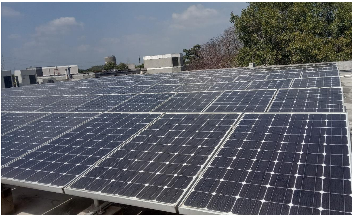
Solar Panel Installed at Admin Block of the campus.
