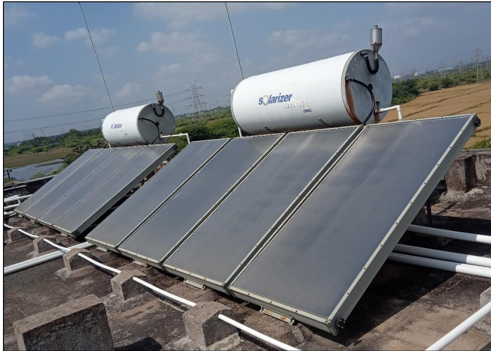
Solar Water Heater installed Hostel Blocks
