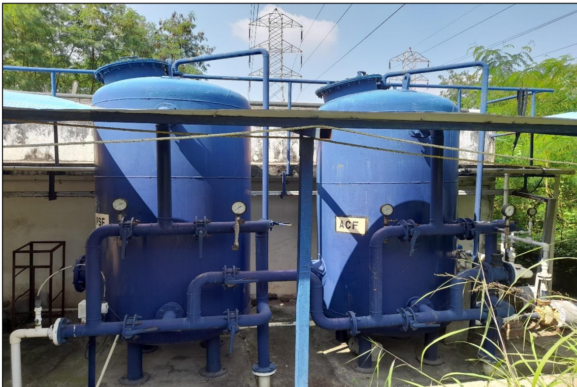
Pressure Sand Filter & Activated Carbon Filter
