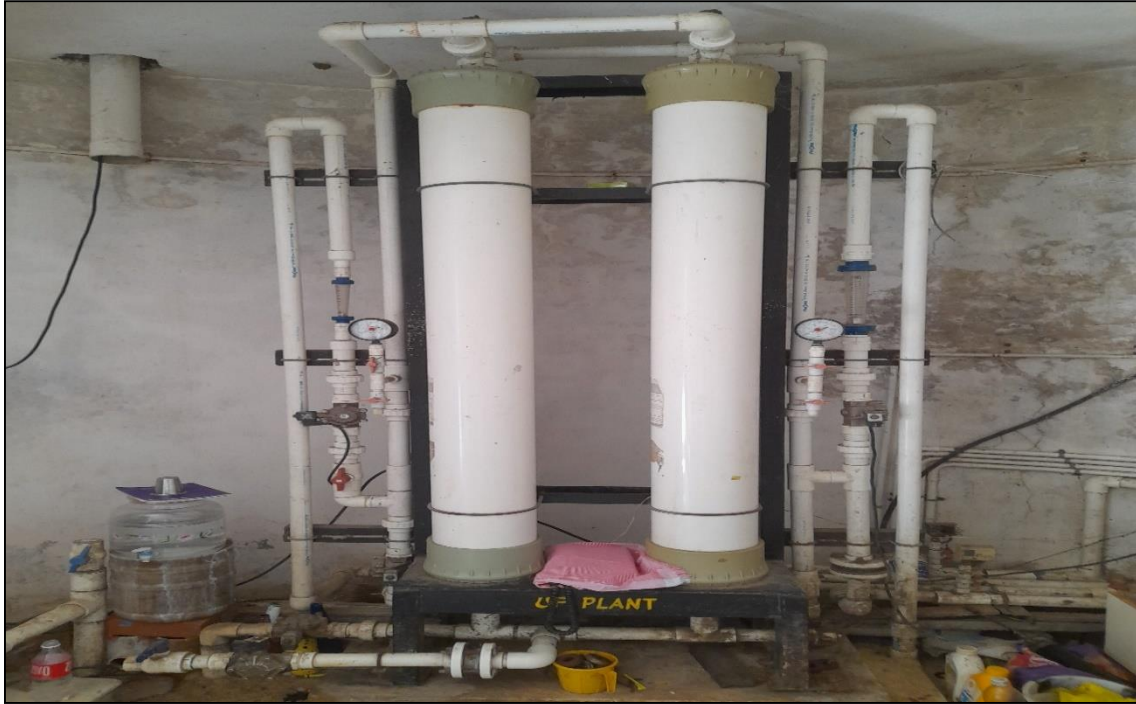
Ultra Filtration Plant
