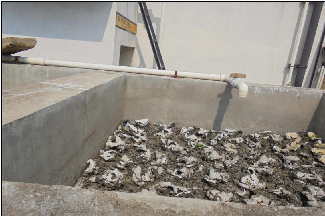
Sludge Drying Bed
