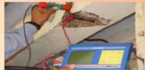
MEASUREMENT OF CORROSION
